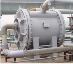
Waste Water Cooler
